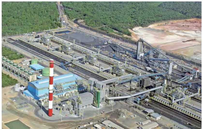
Coke oven gas recovery power plant for Brazil
