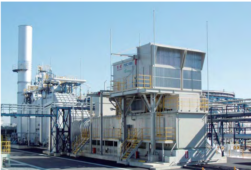
15.9 MW gas turbine cogeneration system for MC Shiohama Energy Service Corporation
