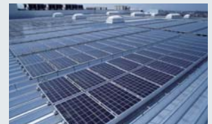
The photovoltaic power generation equipment installed at the KPM (Kawasaki Precision Machinery Ltd.) main plant
